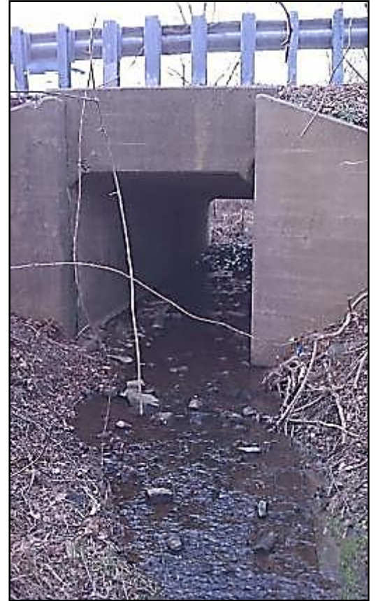
Figure 10 Cattle Tunnel that can be used as trail connector. Note the flooding after heavy rains.
